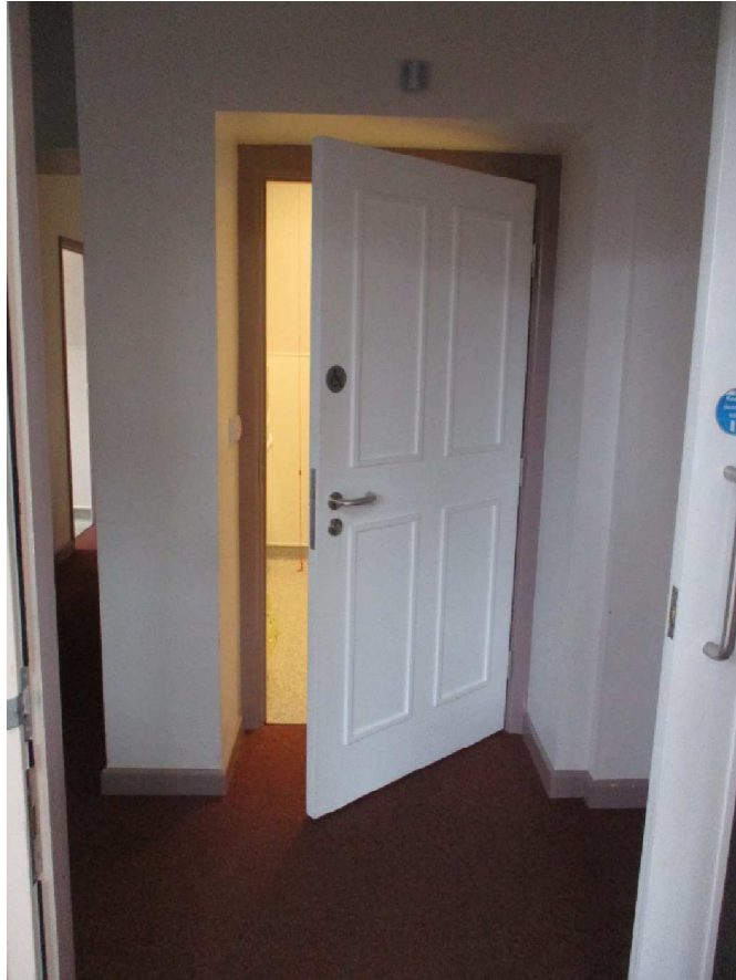
Photo 20 – Restricted access adjacent leading edge to Accessible WC door.
