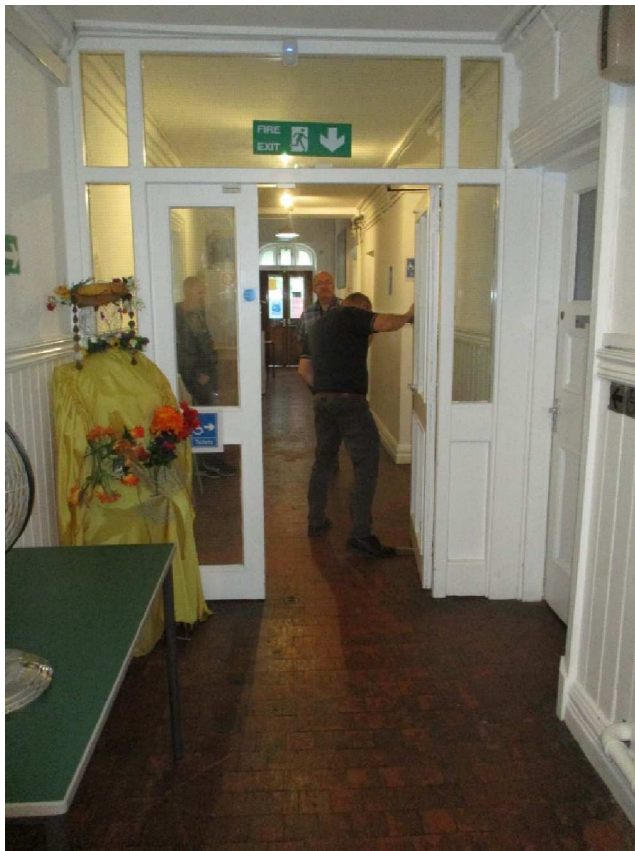
Photo 12 – Cross corridor door, not held open.
